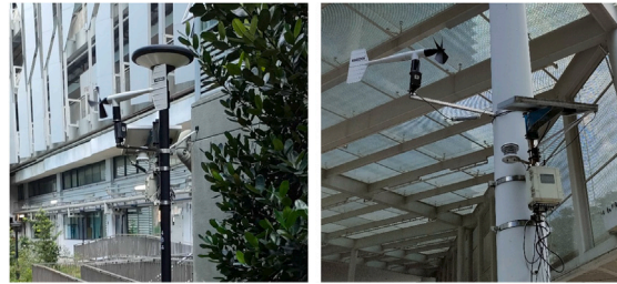
Fig. 3. Equipment for weather stations.
